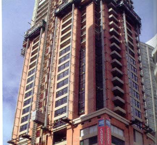
16 single mast units surrounded the building. Bridge units connected the tower units. Outriggers extended platforms into set back corners. System supported a total capacity of 96,000 lb.
